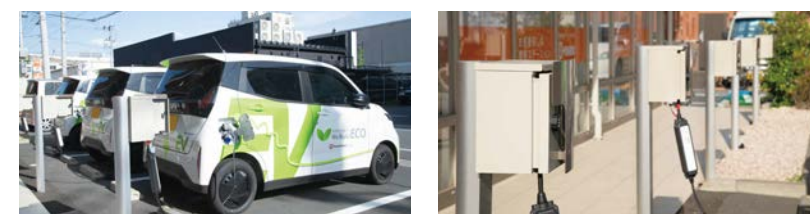
EV charging stations
